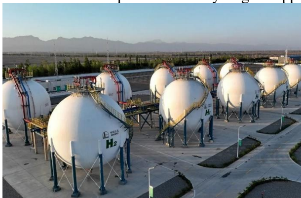
Fig. 1 Hydrogen storage tanks at Sinopec's Kuqa project, Xinjiang. (Photo: Sinopec)
