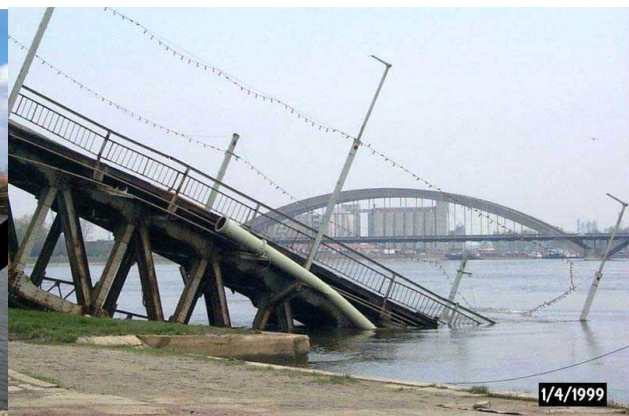
Fig. 2 Varadin Bridge on April 1 st , 1999 (Zezelj's bridge is seen in the background)
